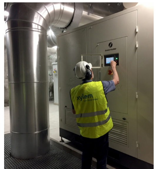
Xylem employee assisting in startup of MAX600 (400kW) blower.
